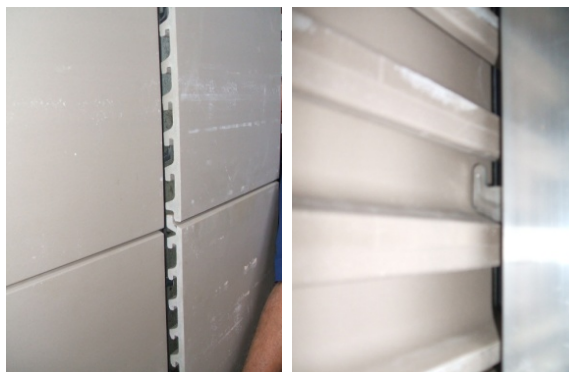
Photo 9. Relative rotations and displacements between facades tiles at maximum drift of 3%
